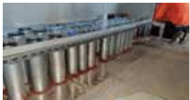
Multiple penetrations (riser banks)
